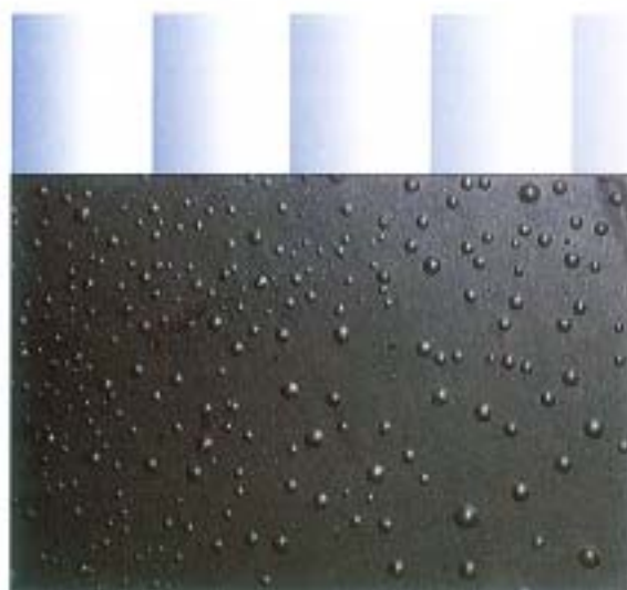
Blistering, such as that shown in the rubber lining at left, has a variety of causes, including proprietary additives in the lining and steam cleaning. Courtesy of Jim Molnar, Union Tank Car
