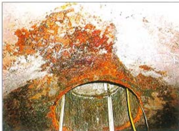
Federal regulations require periodic inspection of lined cars that carry corrosive materials. Molten sulfur service is among the most corrosive environments for railcars. Coating failure at the manway is shown here.
