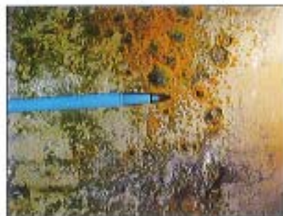
Gathering data on lining performance, like the failure and pitting above, is crucial to improving long-term protection.
